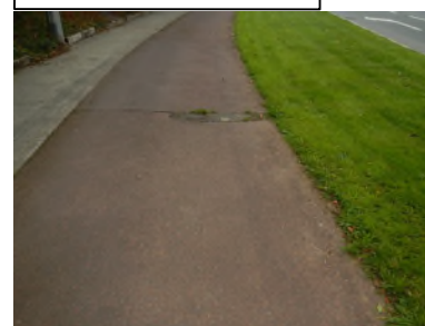
Poor pavement condition
